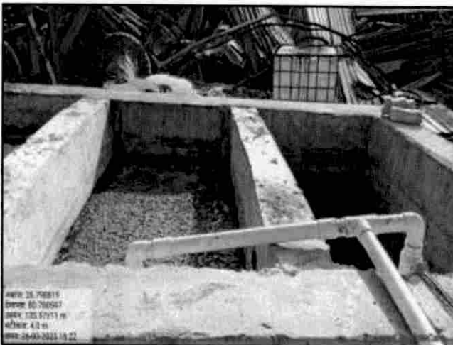
Settling and Sludge Tank
