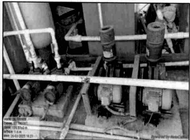
Pump and Blower
